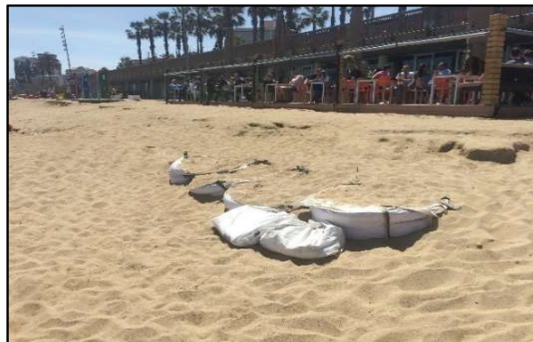
Figure 12. Sandbags placed by the owner of the restaurant Xup! Xup! to protect the beach from the significant retreats of the shoreline
